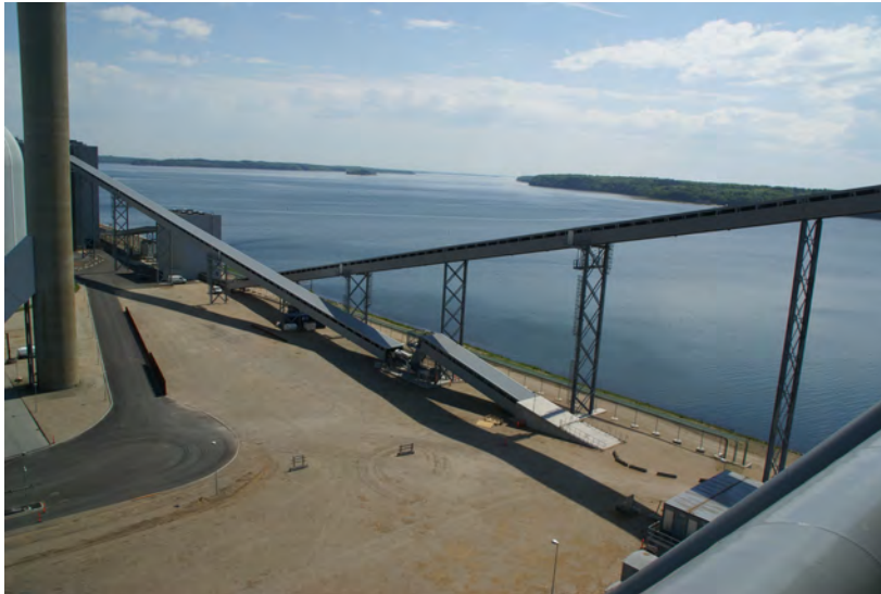
Total 1,5 km Conveying system
