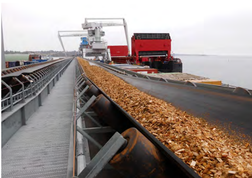
2 x 1400 m 3 /h Conveyors upstream screening building
