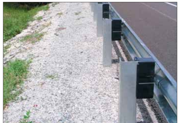
Steel block failure
