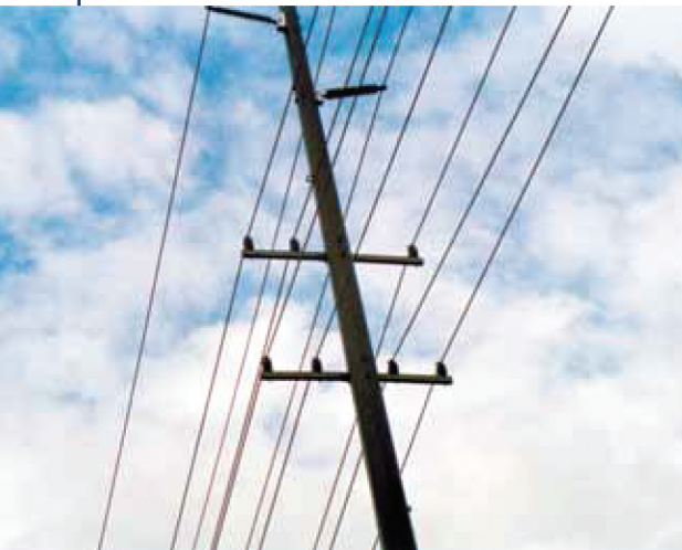
477 ACSR under build project, 14' Lewtex arms
