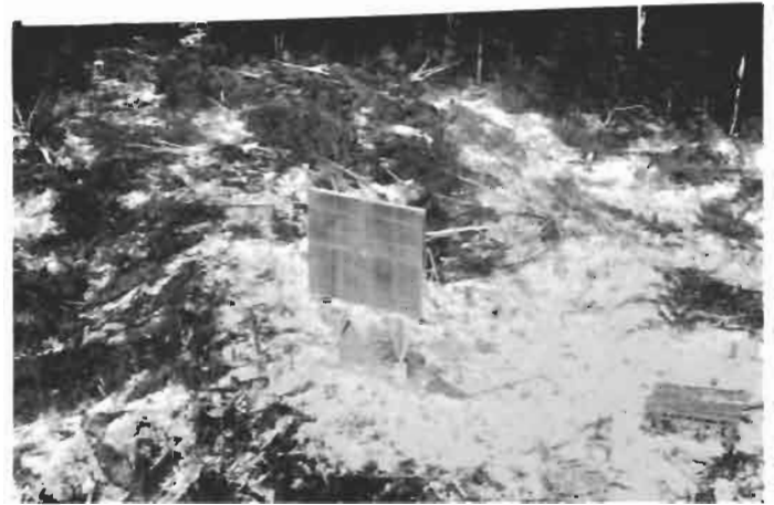
A 16x20 passive repeater is installed in the path between La Tuque and Beaumont.
