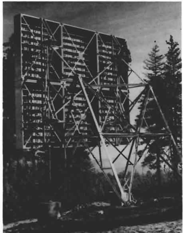
Front and back views of a 20 x 24 passive repeater.
